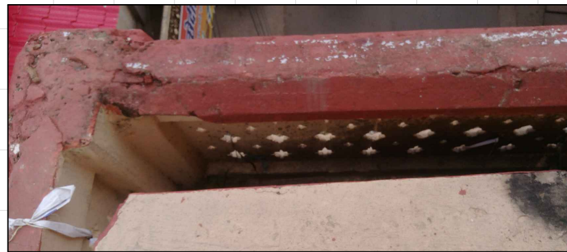
CRACKS ON PARAPET, DAMAGED ELEMENTS, FLAKING OF PLASTER
