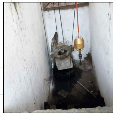
DAMAGED OLD CLOCK, DAMAGED SLAB, DEBRIS
