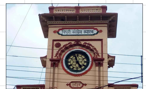
FLAKING OF PLASTER AND DAMAGED BANDS
