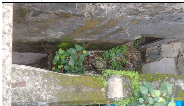
MICROBIOLOGICAL GROWTH ON PARAPET, DAMAGED ELEMENTS ON PARAPET, CRACKS, VEGETATION GROWTH
