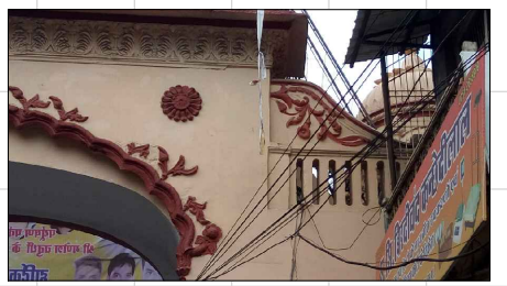
MISSING ELEMENTS ON THE CUSPED ARCH AND DAMAGED ELEMENTS ON THE PARAPET
