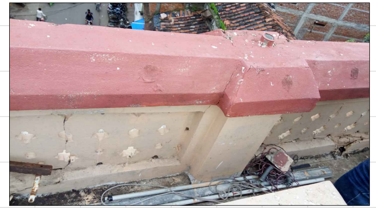
CRACKS ON THE PARAPET
