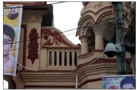
DAMAGED PARAPET AND BANDS WITH SOME MISSING ELEMENTS
