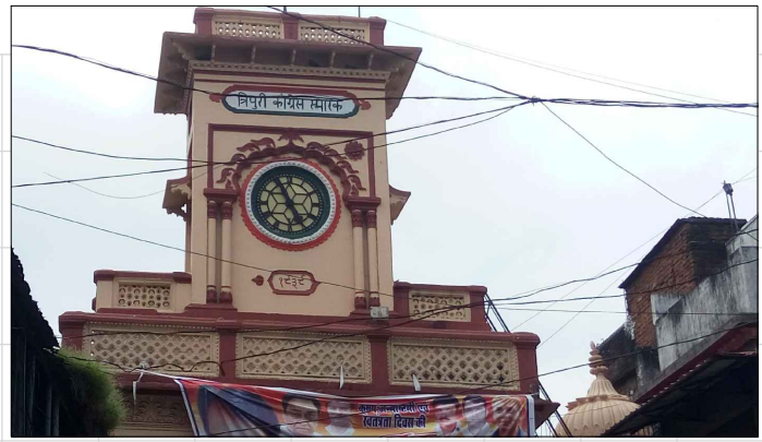
MISSING AND DAMAGED ELEMENTS, CRACKS ON THE PARAPET
